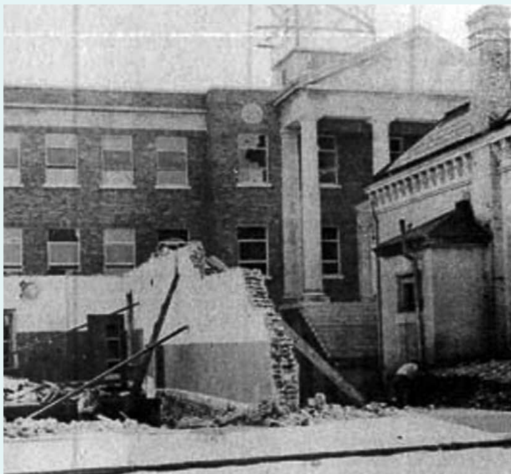
This photo shows the courthouse used from 1872 to 1939 being torn down as the new one is being constructed behind it.
